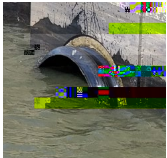
Figure 1 - Recess in anular concrete at OF-00X
