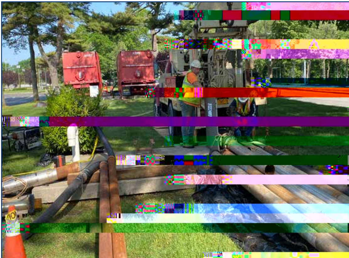
A down-hole rig is used to access the existing remedial extraction well for maintenance and cleanout.
