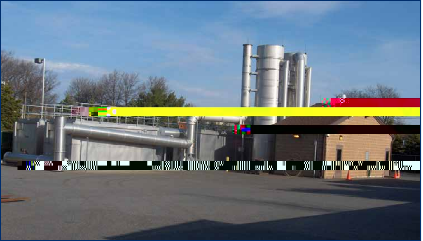
On-Site (OU1) Groundwater Treatment System
